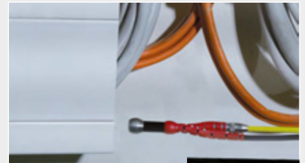
Shafts and underfloor ducting
